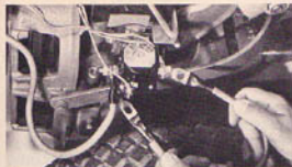
(Photo 1/27) Touch cable to right and center posts.
