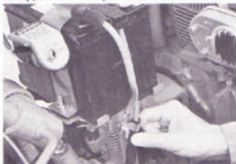
(Photo 39) Attach negative (-) cable and clamp.
